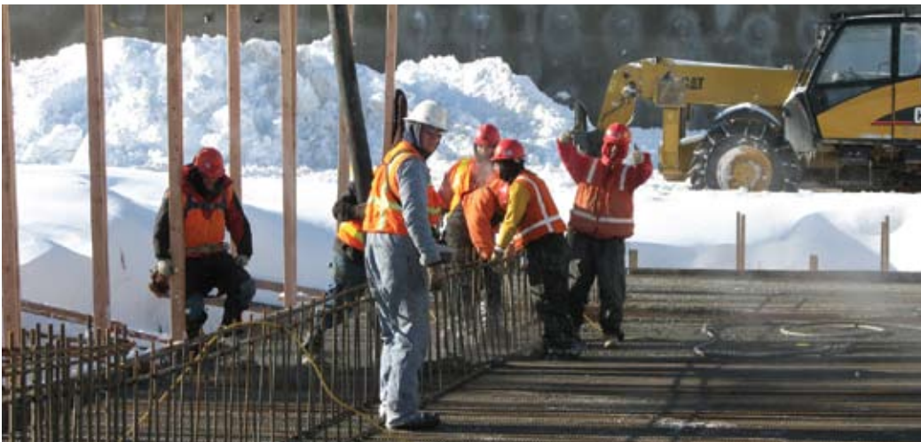
Cold weather offers challenges to concrete-pouring crews, like this one in Park City, Utah.
