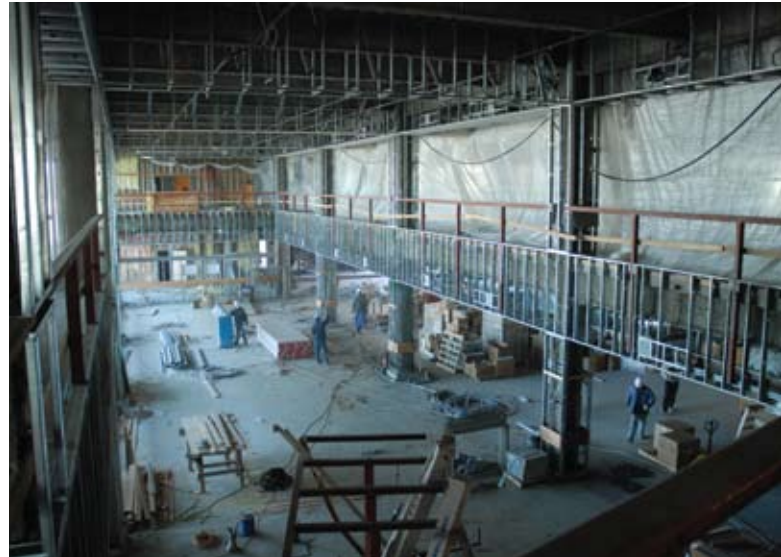
The Utah Valley University Library is built upon a concrete pour of 3,200 cubic yards – a record for Layton Construction.
